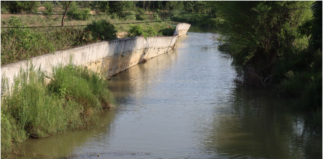
Photo 59: Awaiting disaster: the incomplete embankment in Singhe river
