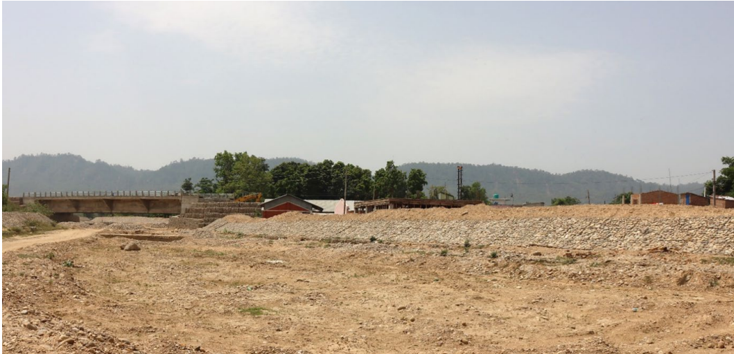
Photo 17: Ongoing bridge construction in Mahadewa River with the nearby houses below the riverbed
